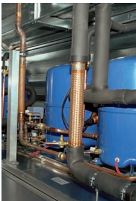
Compound connexion with four reciprocating compressors
