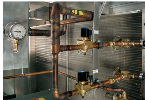
Cooling piping provided by customer technical changes
