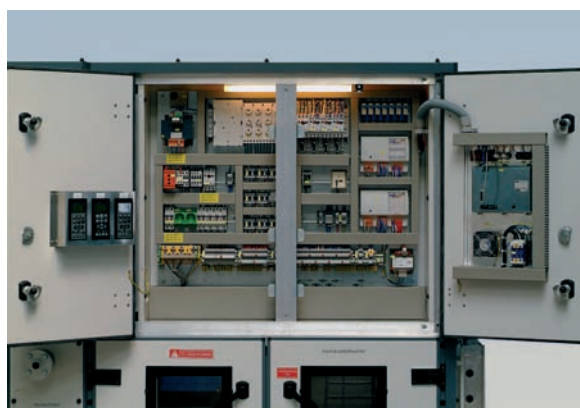
control cabinet with DDC module
