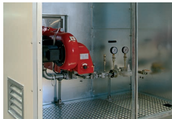
group of controllers for combustion chamber
